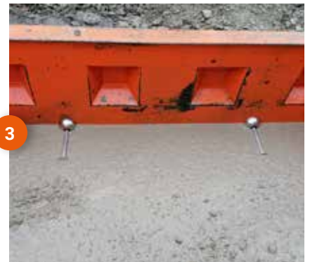
3 The anchor is cast in its entirety, be careful when vibrating the concrete
